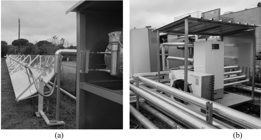
Figure 5. The solar powered ORC, (a) solar collectors (b) ORC prototype [28]
