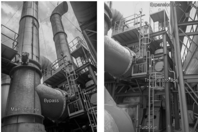
Figure 6. Flue gas-Heat exchanger and modified chimney [47].
