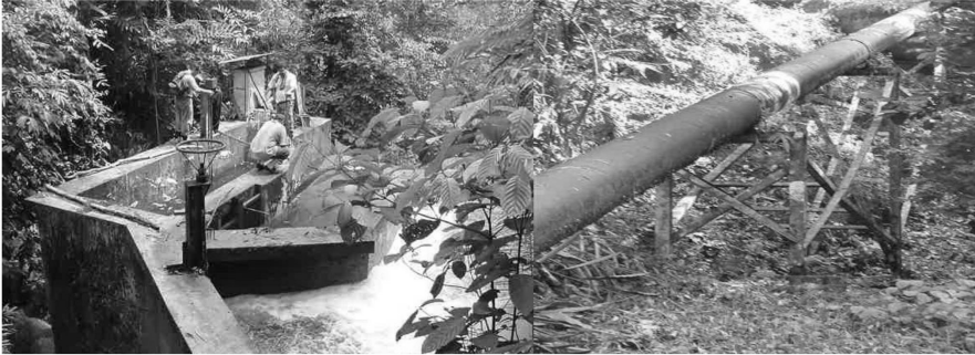
Figure 2: Control Water Valve and Steel Type Penstock
