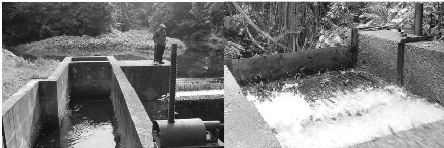
Figure 1: The Intake of River Water and Automatic Racking System
