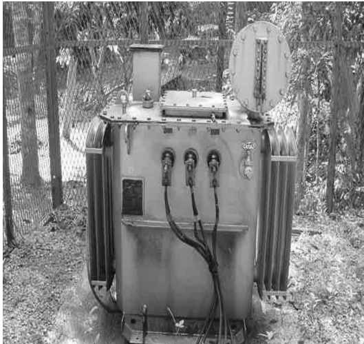
Figure 4: Transformer to Step Up the Voltage
