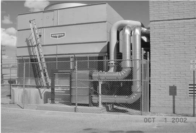
Figure 2. 1,700-Ton Tower Free-Cooling System
