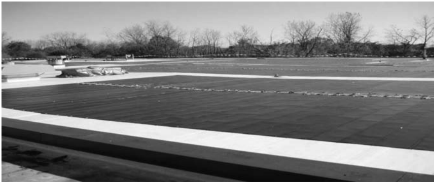
Figure 1. View of thin film PV mounting arrangement
