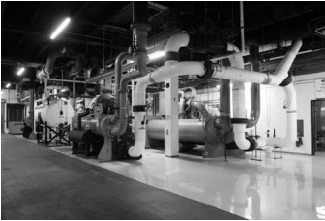
Figure 1. Park City Central Utility Plant
