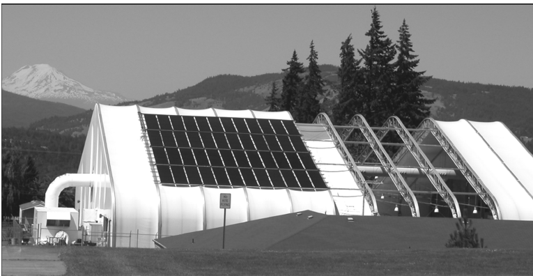
Figure 1. Solar System and Open Pool Roof. (Photo Credit: Brent Gunderson, Gen-Con Solar)
