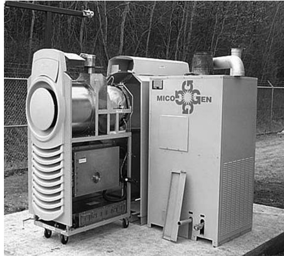
Figure 4. Internal View of a Microturbine
