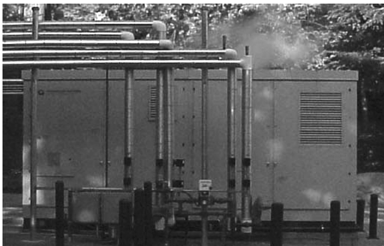
Figure 13. 200 kW Fuel Cell
