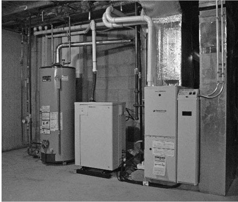
Figure 19. The Micro-CHP System
