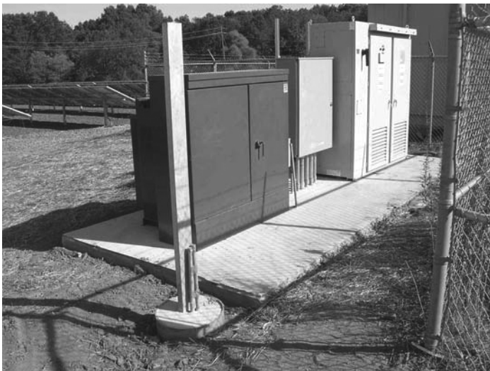
Figure 4. Satcon Inverter and Transformer
