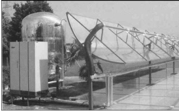
Figure 1. Solar Thermal Collectors
