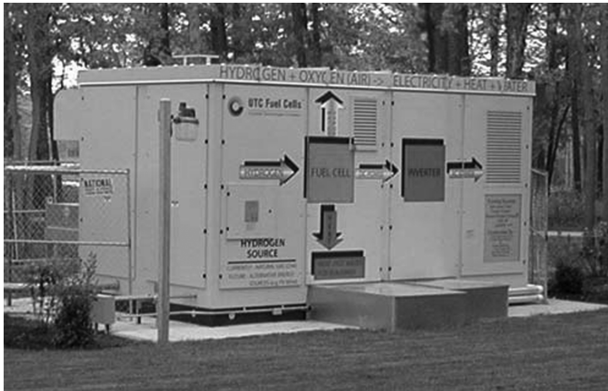
Figure 1. PureCell™ Model 200 Installation, Stockton College, NJ
