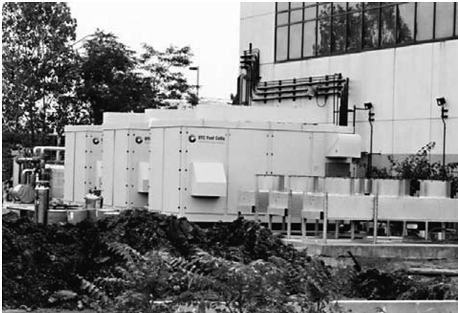
Figure 6. NYPA Wastewater Facility, Hunt's Point, NY
