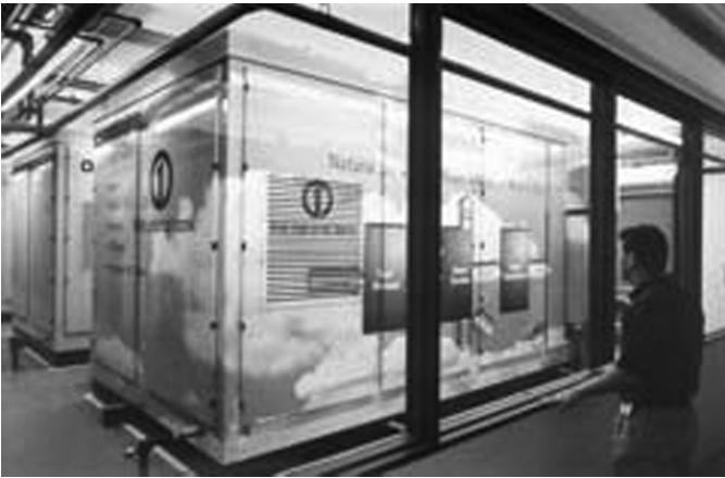
Data Processing Center
