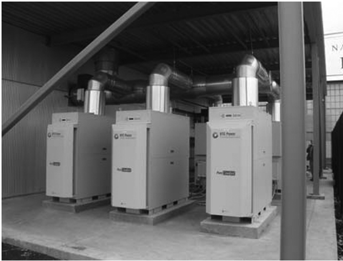
Figure 3. Pure Comfort™ Trigenation Installation at Aviator Sports and Recreation, Brooklyn, NY
