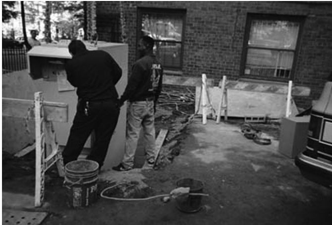
Figure 2. Microturbine Installation at the Clinton Hill Apartments, Brooklyn NY
