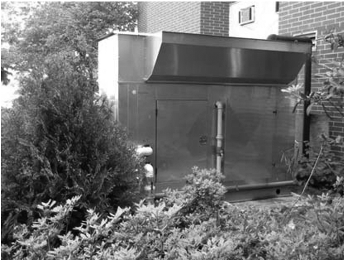
Figure 1. Example of Low Emission Natural Gas Internal Combustion CHP System for a Health Care Facility.
