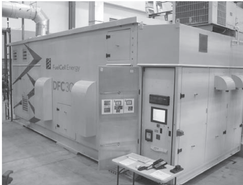
Figure 1. 250 kW fuel cell power plant operating on propane at CTC.
