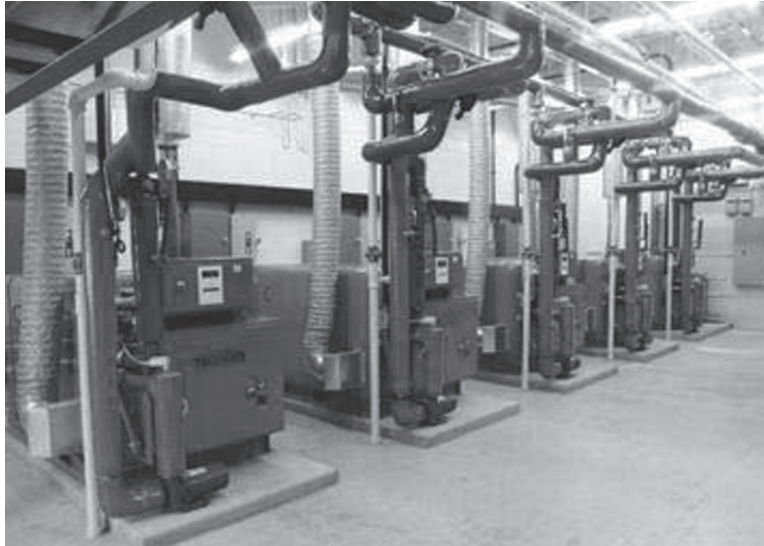
Figure 15. Power Generation Installation
