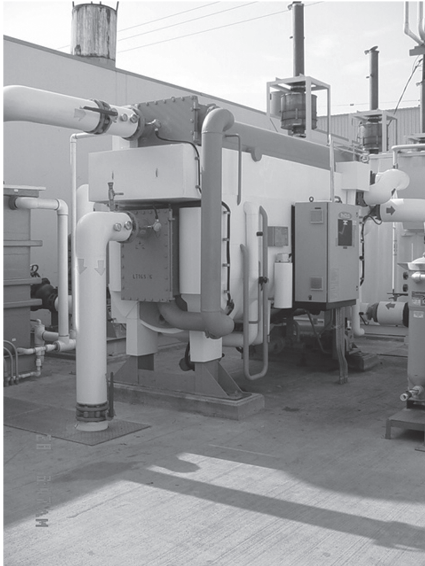
Figure 9. Hot-Water-Driven Absorption Chiller (Photo Courtesy of Thermax)
