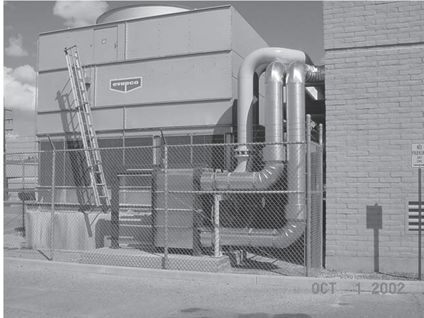
Figure 2. 1,700-Ton Tower-Free Cooling System
