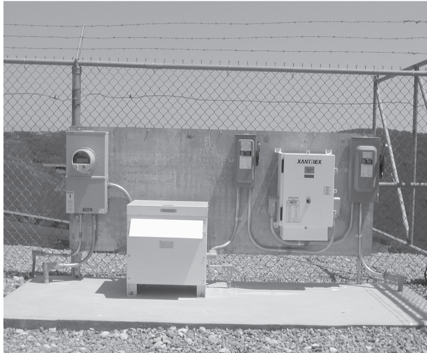
Figure 3. Balance-of-system components, including switchgear and inverter
