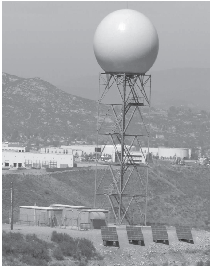
Figure 1. NWS radar site with the 10-kW PV system shown in the foreground
