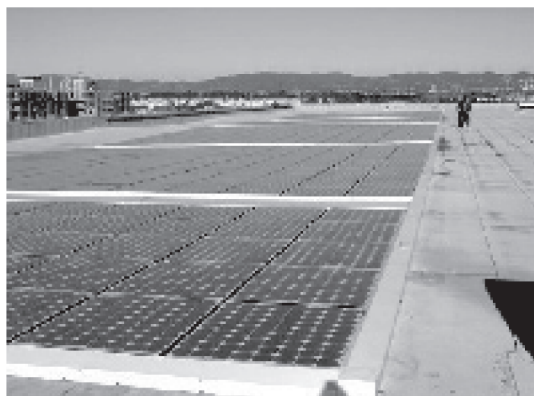
Figure 6. USPS Marina Processing and Distribution Center Array. Source: G. Marsh, PIX 11015
