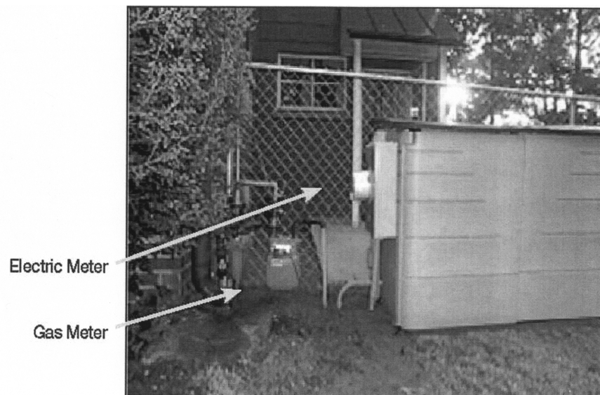
Figure 4. Residential-type Meters to Record Gas Input and Electric Output.
