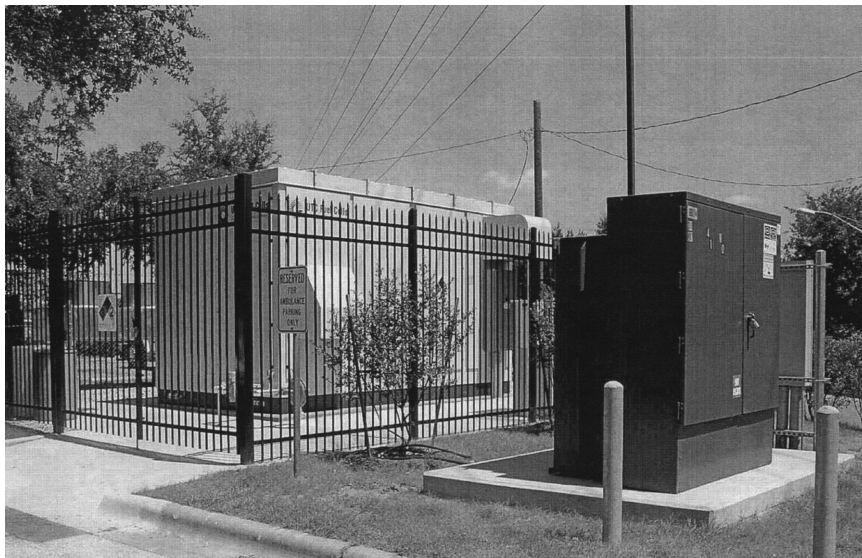
Figure 2. PC25 TM Fuel Cell at RBJ Health Center
