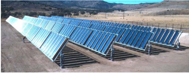
Figure 3. ENTECH SolarRow® Array
