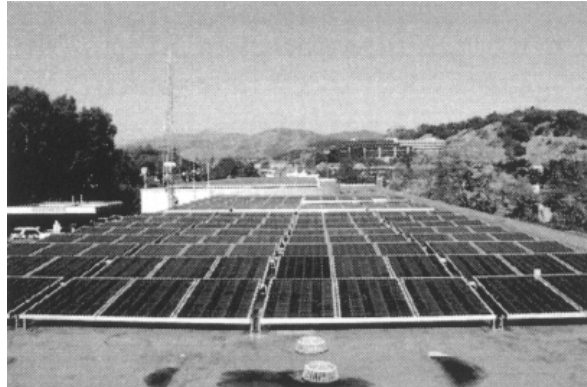
Figure 5. Completed Array Looking North
