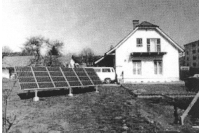
Figure 11. 750 Wp Solar PV Unit
