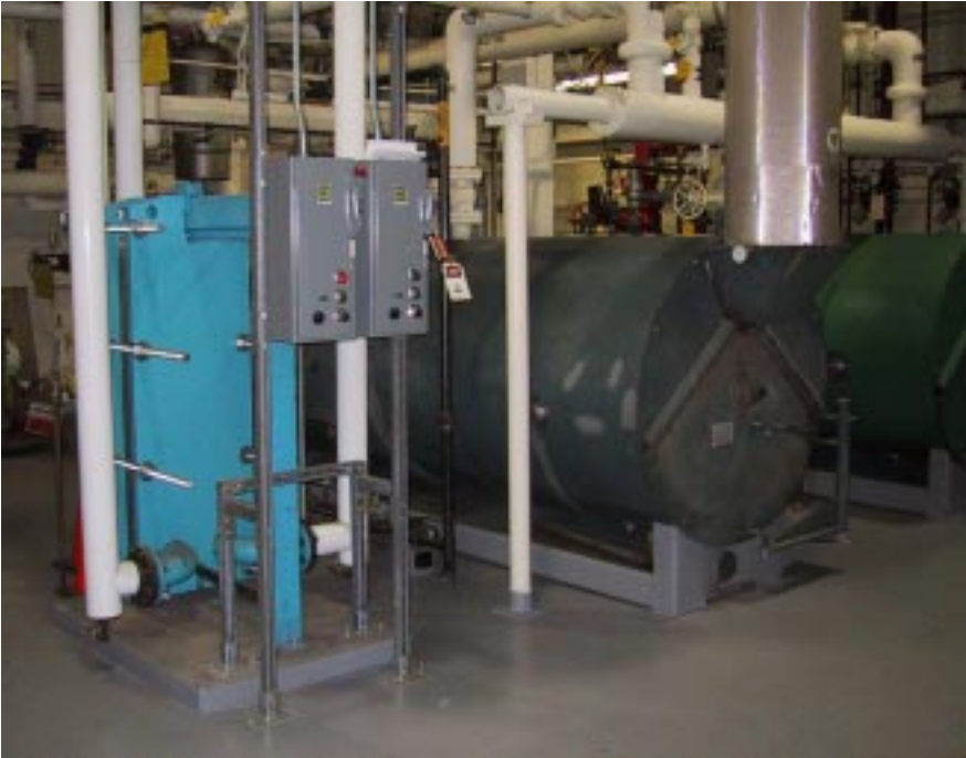
Figure 3. Heat recovered from the fuel cells offsets heat supplied by the boiler system. The boilers were not needed during the winter of 2000-2001.
