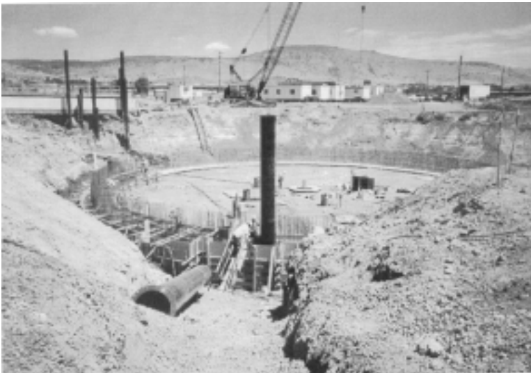
The base of the 110-ft. dia. secondary clarifier, under construction, at the Klamath Falls wastewater treatment plant. Photo: Courtesy IMCO General Construction
