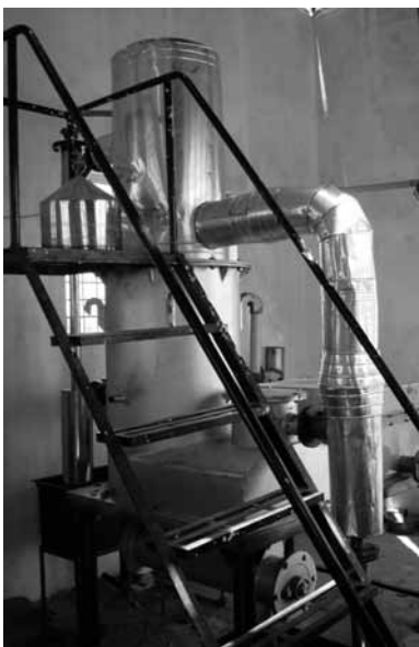
Figure 2. Existing 10 kW Biomass Gasification System (RGTU 2007)
