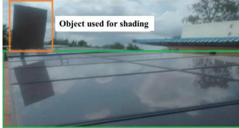
Figure 5 Partially shaded PV modules.
