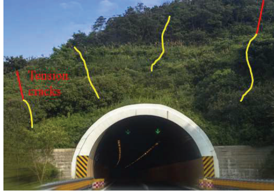
Figure 1 Typical tunnel surrounding rock cracking patterns.
