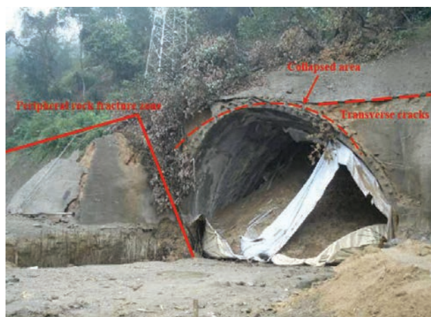
Figure 2 Schematic diagram of the tunnel collapse through the fault activity zone.
