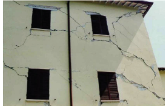
Figure 10 Building damage due to in-plane loading.
