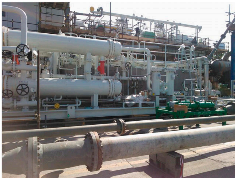
Figure 9. Lube oil plant (courtesy of GE Nuovo Pignone).
