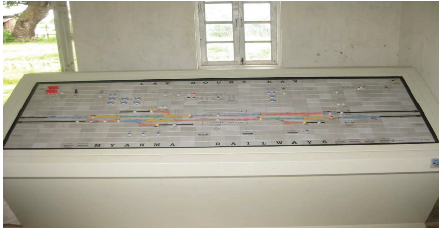
Figure 2 Signaling Panel at IR station.
