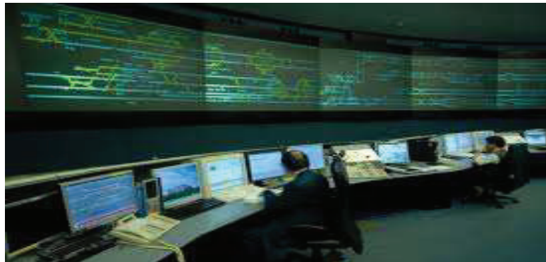
Figure 5 CTC Control Centre at Tundla.
