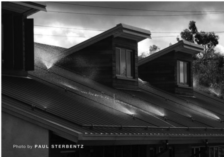
Figure 2. The night sky system which produces chilled water for the building's mechanical systems is shown in spray mode (photo by Paul Sterbezt).
