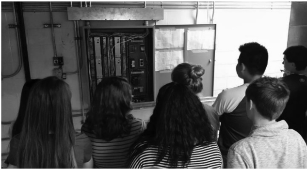
Figure 4. Students viewing building automation circuitry.
