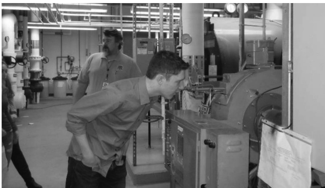
Figure 3. Student viewing the boiler fire tube through the sight glass.
