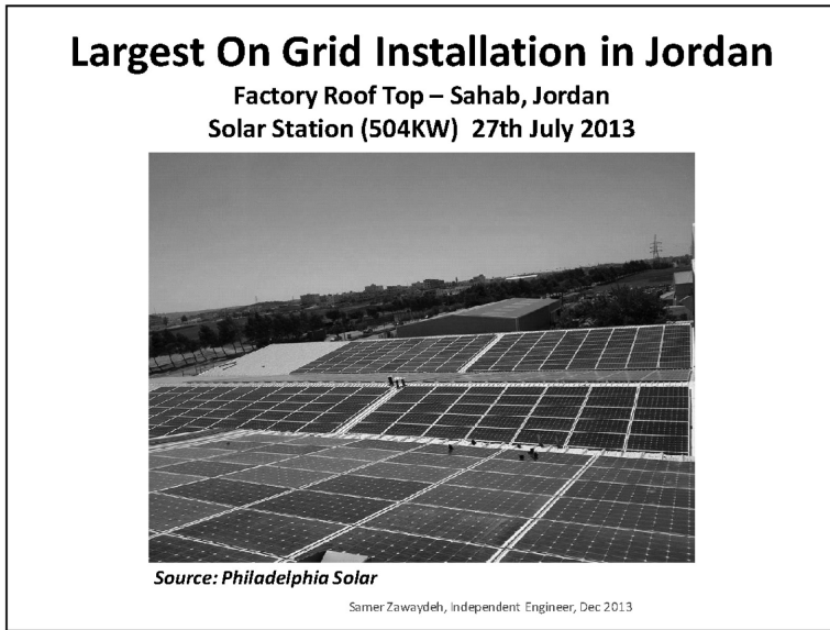
Figure 13: Industrial Rooftop PV Project
