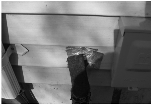
Figure 5. Air conditioner condenser pipe wall penetration, which has been corrected with simple expanding foam and tape.
