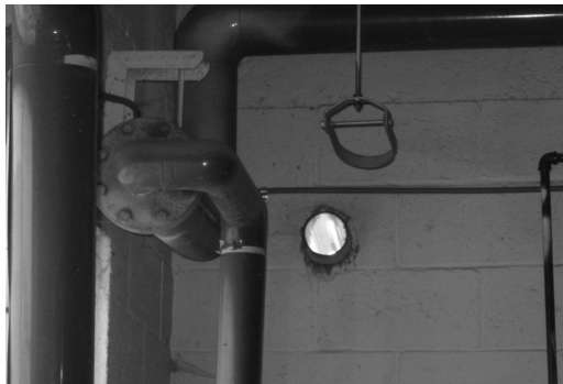
Figure 6. Hole in wall from former pipe wall penetration—never closed off or sealed.
