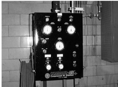
Figure 8. Compressed Air Pressure Controller
