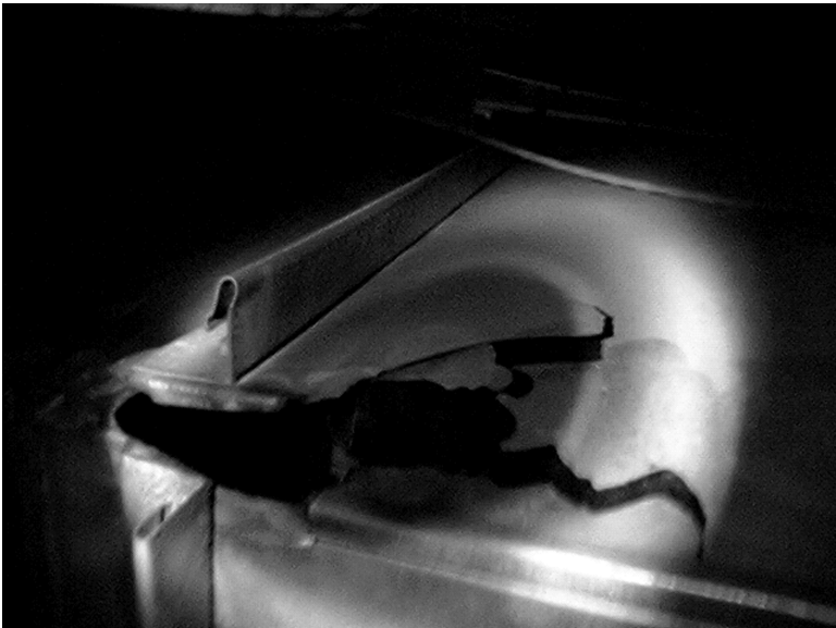
Figure 4. Broken Supply Duct
