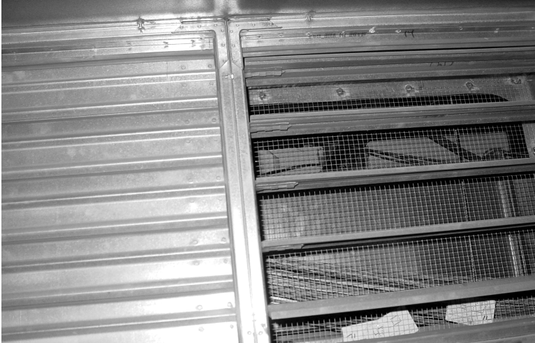
Figure 3. Return Air Damper
